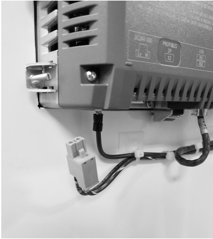
Figure 2.3.1c Power connection removed from HMI.
