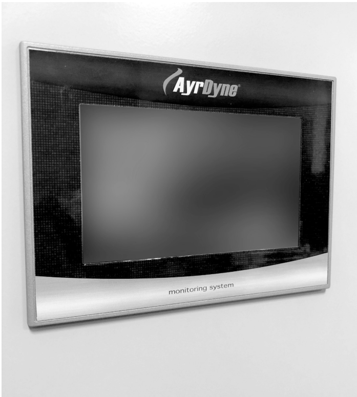
Figure 2.3.1a Front view of HMI.
