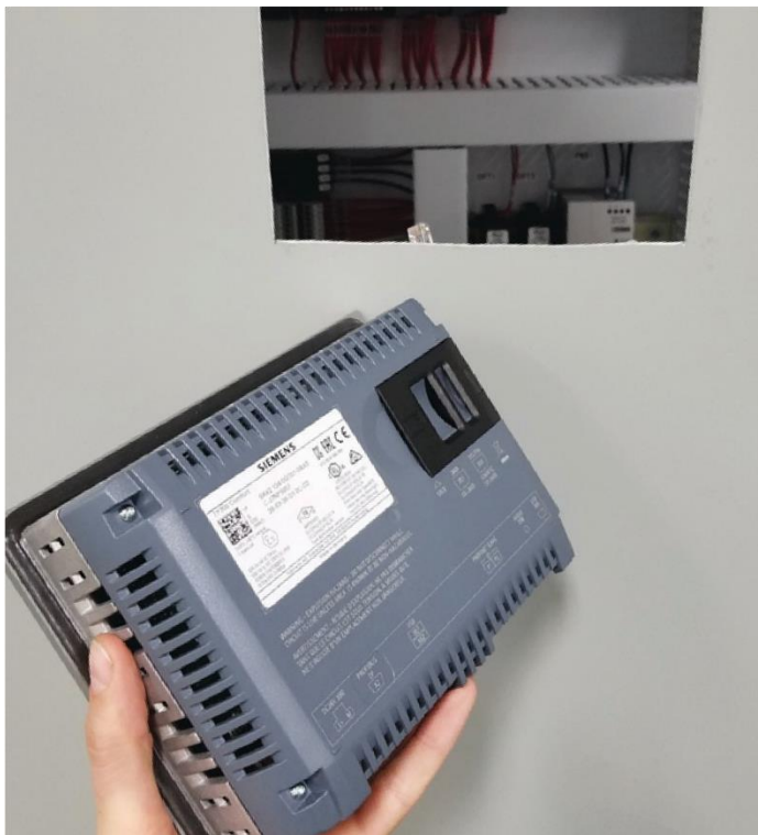
Figure 6 HMI completely removed
