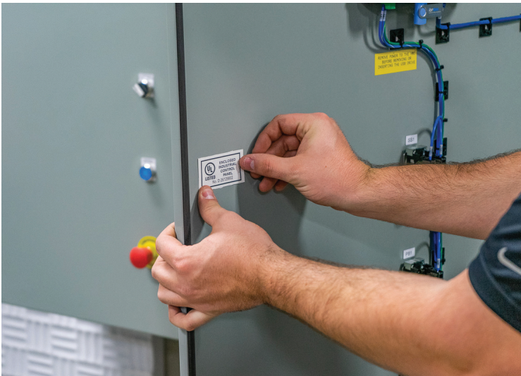
Electrical control panel shop certified for UL508 and UL698A
